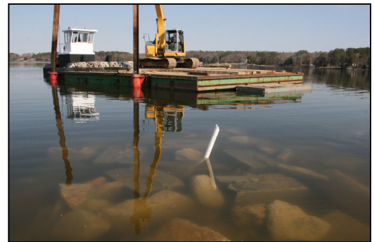
Project contractor Colliflower & Peterson places reef balls in designated locations to construct the 3-D Reef in the St. Mary's River.
