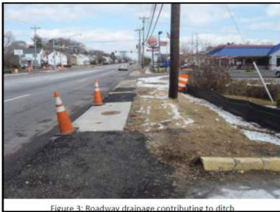
Figure 3: Roadway drainage contributing to ditch
