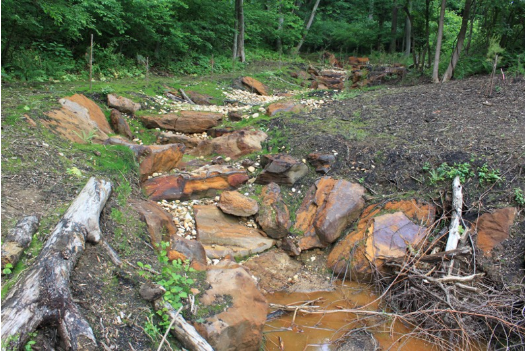
Figure 9. Regenerative Stormwater Conveyance (Underwood & Associates)
